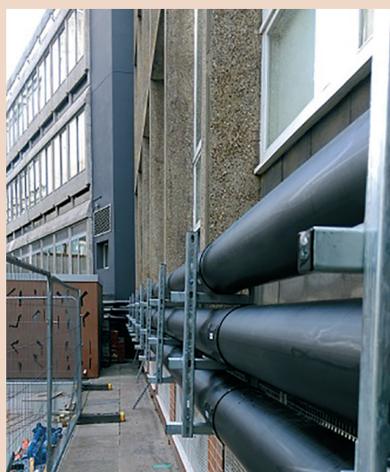
Low diameter plastic pipes have been mounted on the walls of existing buildings to avoid the cost of digging up the roads
