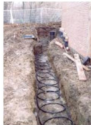
The 'slinky' ground loop being installed in a trench at the National Energy Foundation
