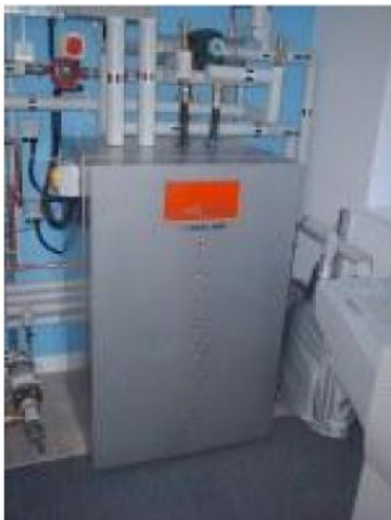
The Heat Pump in the GSHPA offices
